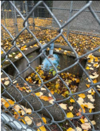
Photo 5: Large diameter upper surface casing. Easton Water District Well #2.
