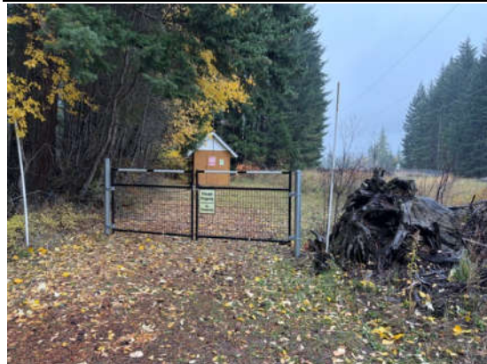
Photo #6: Easton Water District Well #1, AFT-392
